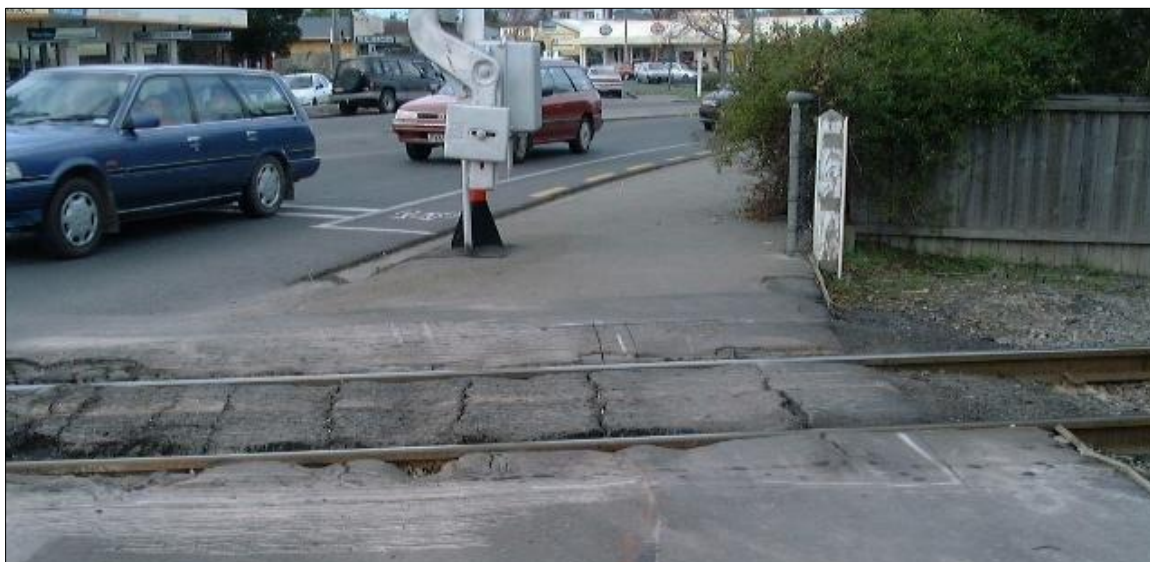
Figure 5-22: Poor pathway maintenance affects the safe available path for many users
