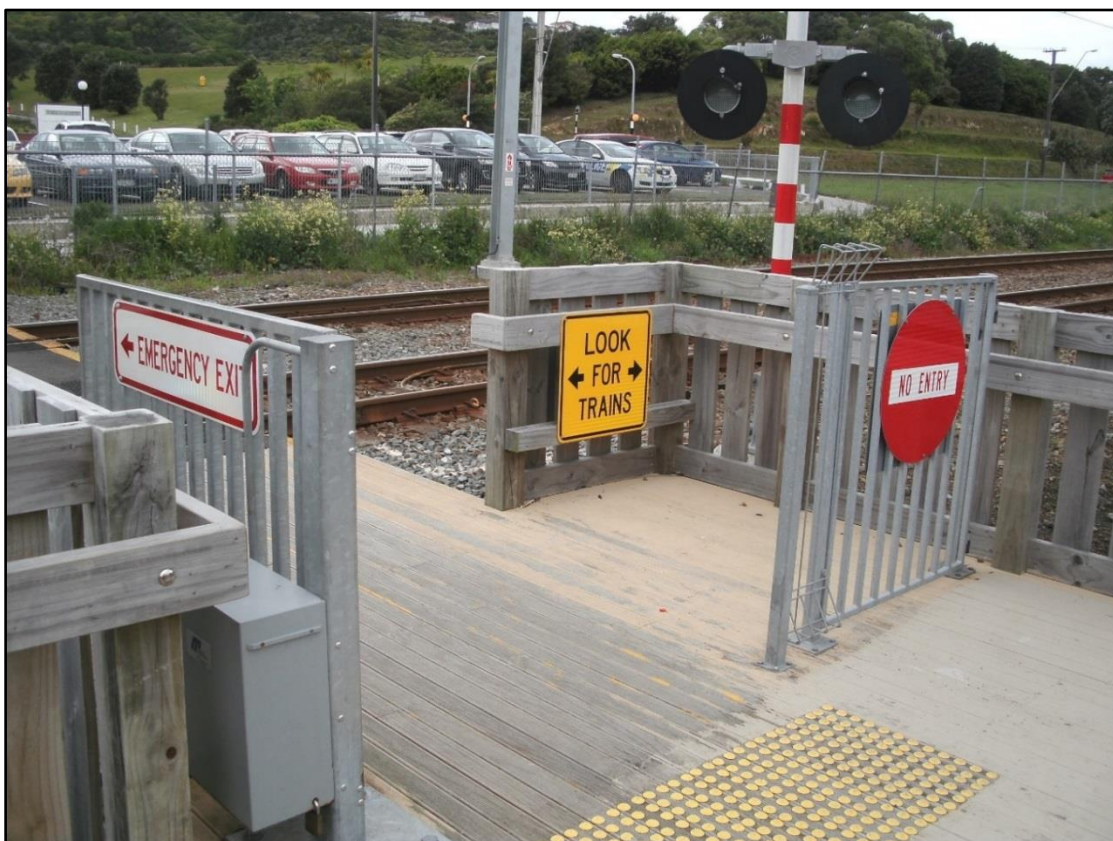
Figure 6-6: Automatic gate, normally open, with emergency exit to the right (Tawa, Wellington)
