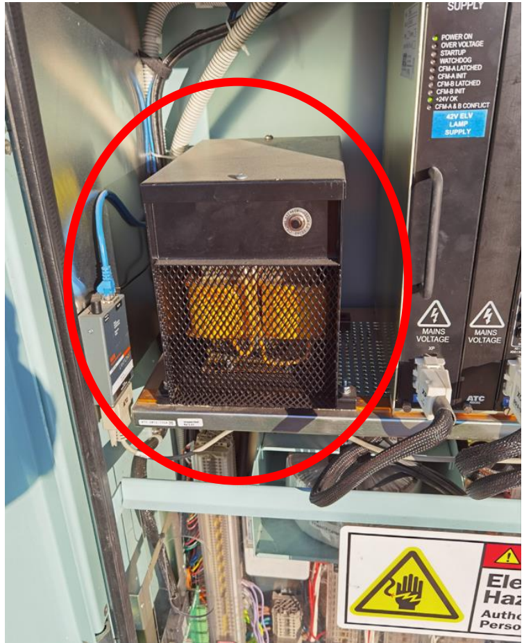
Photo 1 - Step-Down Transformer installed on cabinet shelf
