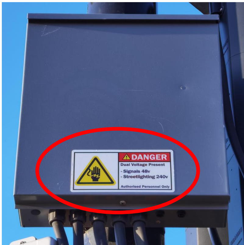
Photo 4 – Labelling Requirement and location on Montrose box
